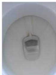
Water scale stains
